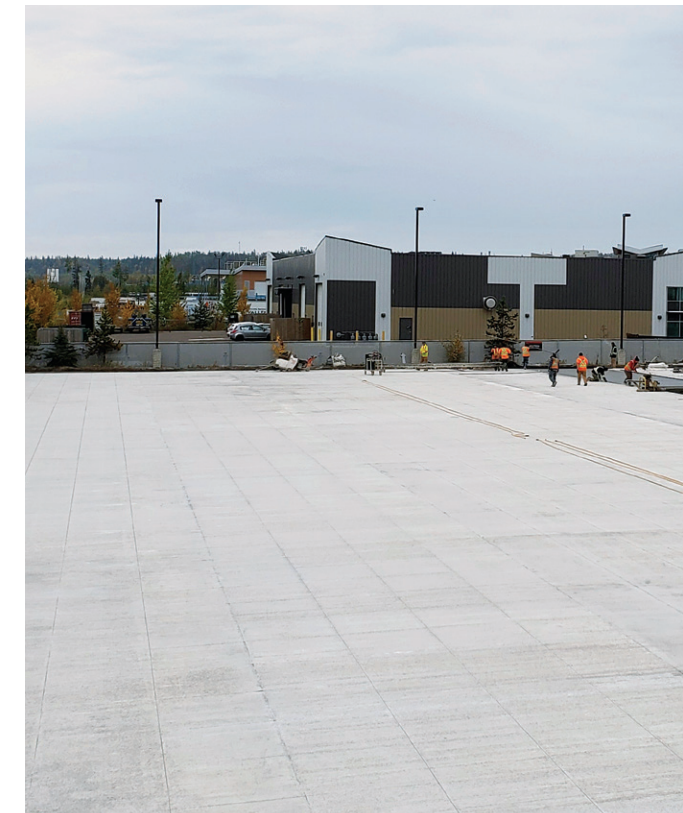
Cummins Fort McMurray Yard Reconstruction 2022 — ACI Awards of Excellence in Advanced Concrete Construction
